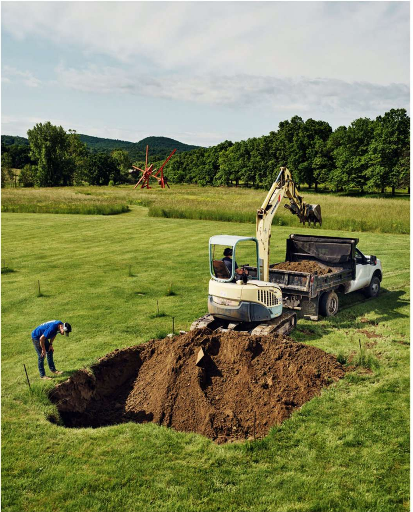
Joel Longinott and Robert Finch dig a hole for a new installation. Mark di Suvero's "Figolu" (2005-11) sits in the background. Thomas Prior for The New York Times
